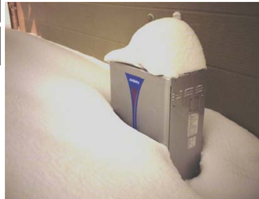
Fig.5 Photo of the system installed
